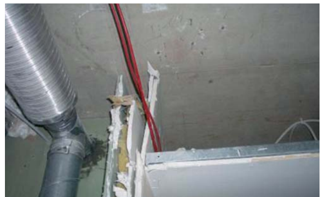
Abb. 8c: ... fehlende CE-Profile Figure 8c: ... missing CE profiles
