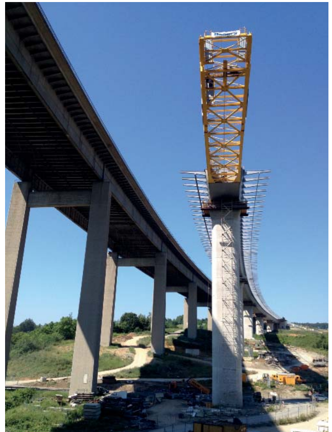
HEIDINGSFELD VIADUCT, an incrementally launched composite bridge cantilevering up to 120 m during erection near Würzburg along Highway A3.
