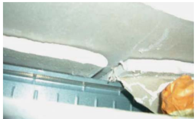
Abb. 8b: ... fehlende Verspachtelung ... Figure 8b: ... missing body filler, ...
